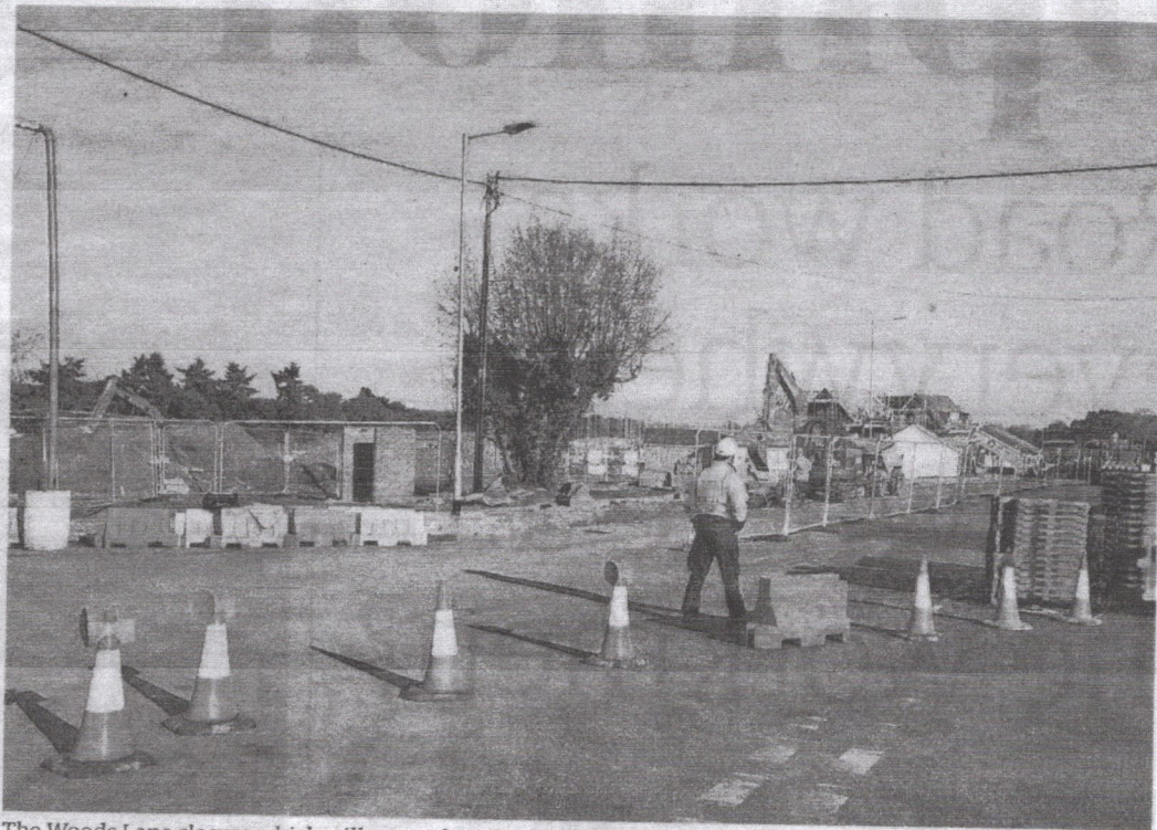
The Woods Lane closure which will cause chaos in the Woodbridge and Melton area for the next few months.
