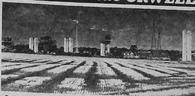
By the autumn of 1980, work on the west bank piers was well under way. To support them, foundation piles were driven, up to 131 feet below ground-level.
